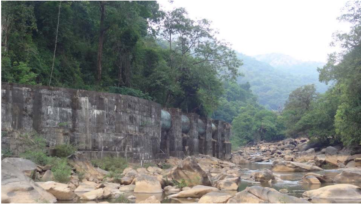
The penstock pipe diverting river flows from the weir to the powerhouse. Such linear structures are insurmountable barriers and drastically impede the movement of wild animals such as elephants.
